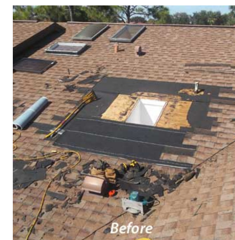
A roof repair program is a part of the NRSA plan
